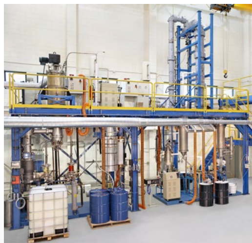
Pope Toll Processing & Pilot Facility, Saukville, WI
